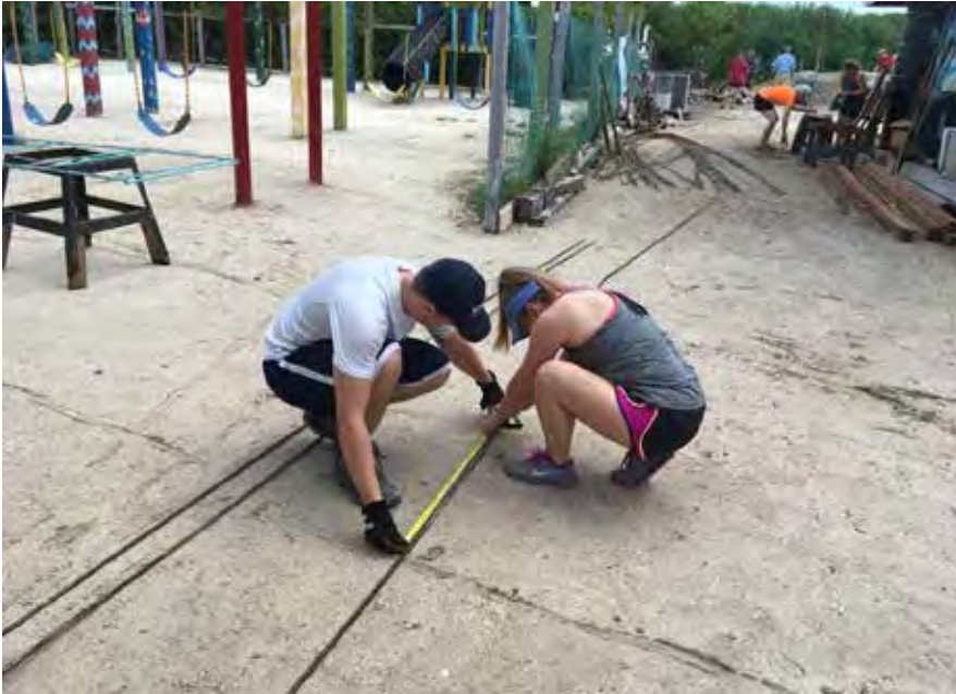
Matt Albritton and Laura Fleming measure and straighten rebar that will be cut and welded into bike racks.
