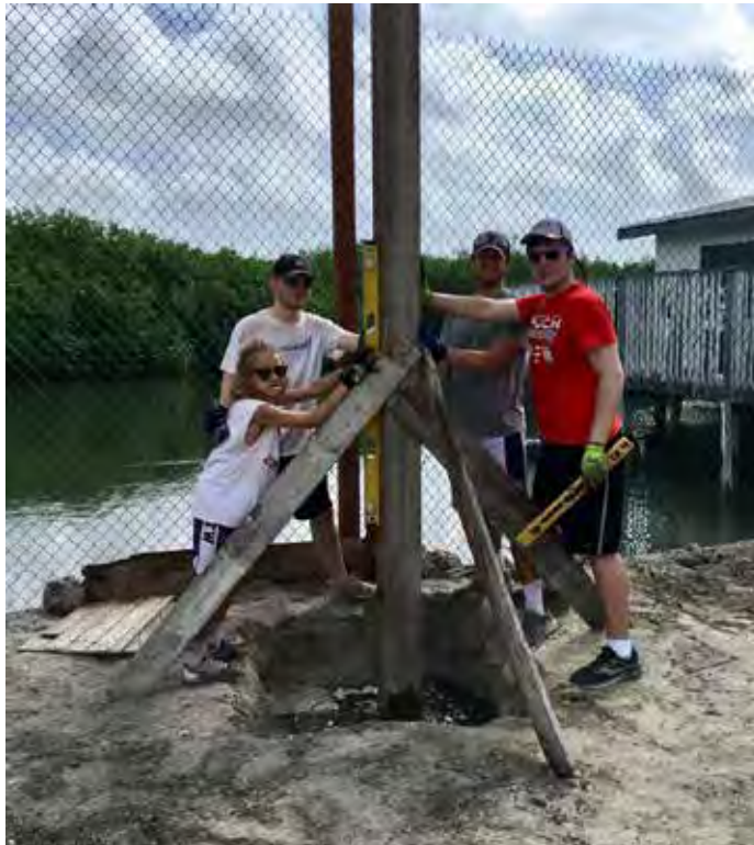
Christian Johnsen, Ben Albritton, Caleb Albritton and a youth missionary installed this new post.
